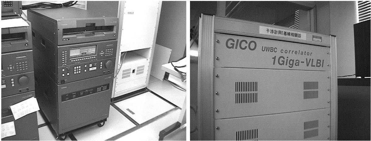
Figure 2. Completed Giga-bit recorder (left) and UWBC-GICO experimental correlator (right)
