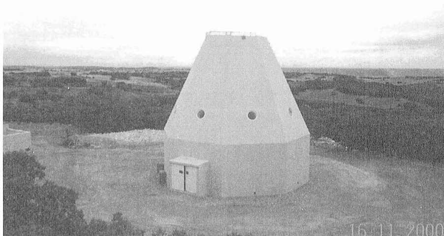
Figure 2. Status of the construction of the new 40 meter radiotelescope of OAN at Yebes (Guadalajara, Spain). The finished concrete pedestal is shown.
