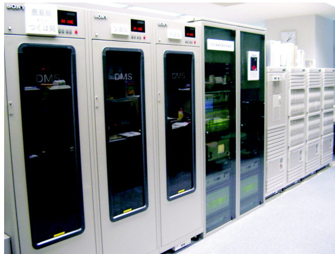
Figure 1. K-4 (KSP) correlation devices at Tsukuba VLBI center. The three boxes on the left are automatic tape changers. In each, a playback recorder is installed. There are two racks at the center. The three correlators, system controller and other devices are stored in the racks. On the right, there are workstation and disk array to run correlation software and SOLVE.
