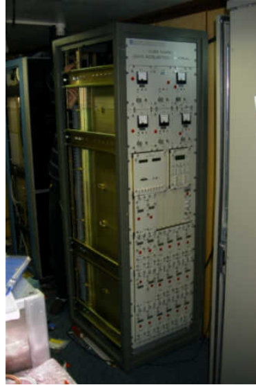
Figure 2. DAR after the finish of MkIV upgrade
