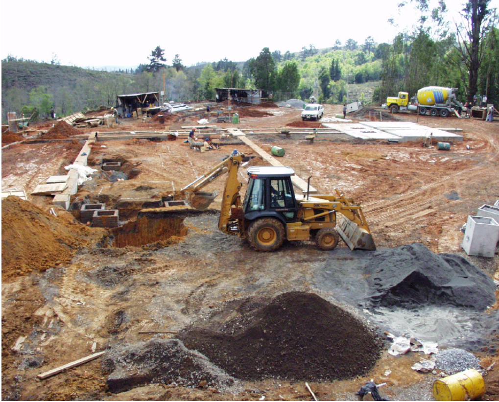
Figure 2. September 7, 2001. TIGO platform with foundations for five containers (left) and the radiotelescope (right). Two of the reference pillars for controlling local site stability by local geodetic surveys can be seen at the far left side and next to camion with concrete at the far right side. In the foreground begins the excavation for the SLR-monument.
