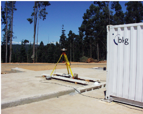
Figure 3. January 24, 2002. GPS measurements are carried out over the central marker for the TIGO radiotelescope. The measurement served for the orientation of the platform and the a priori coordinates of TIGOCONC.
