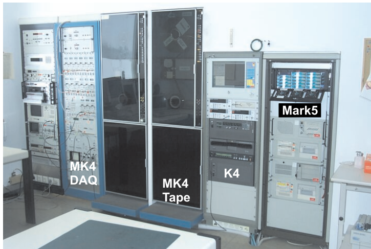
Figure 1. VLBI Data Acquisition System Wettzell.
