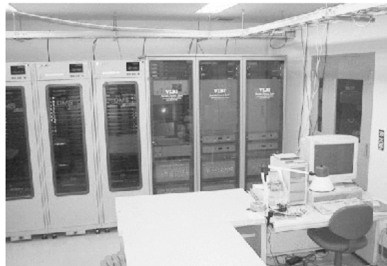
Figure 1. Operation room of KSP correlation system
