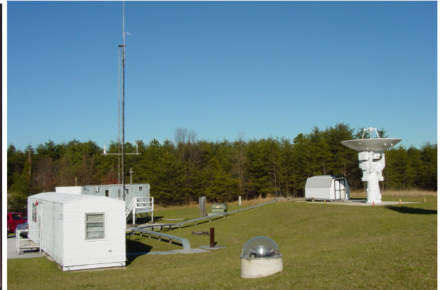
Figure 2. New permanent MV3 antenna.
