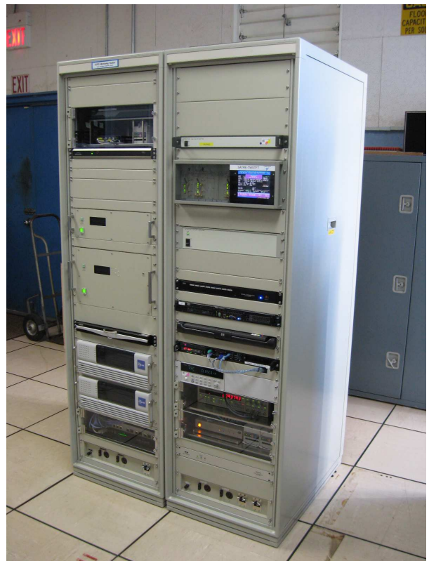
Figure 4. QZSS/TWSTFT equipment racks.
