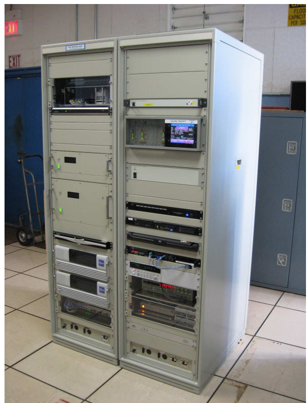
Figure 4. QZSS/TWSTFT equipment racks.
