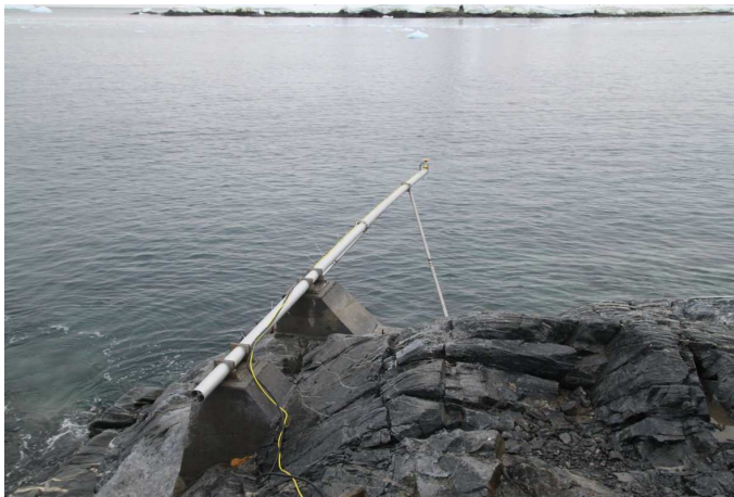
Figure 2. The new radar tide gauge which was installed in 2011.
