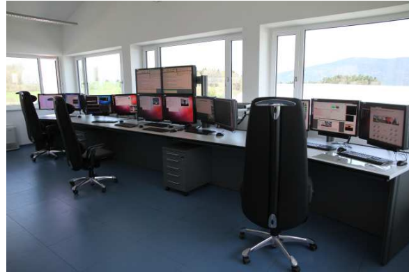
Fig. 4 The new control room and Data Center in the Twin operations building.
