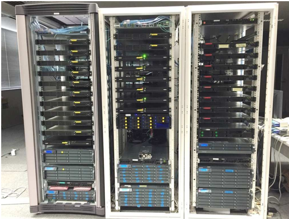
Fig. 2 View of the existing data processing servers.
