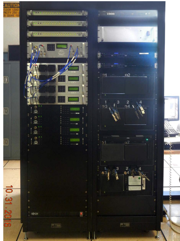
Fig. 4 Signal Chain backend sub-system as deployed at KPGO control room.
