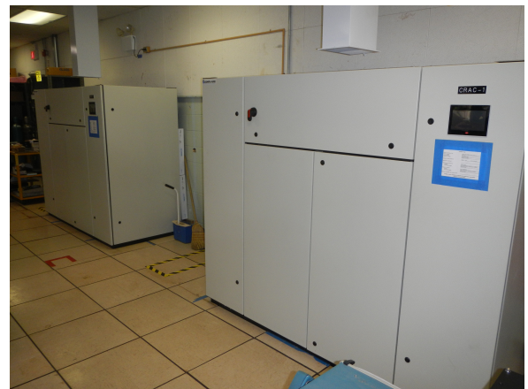
Fig. 3 Newly installed HVAC system for KPGO Operations Building.
