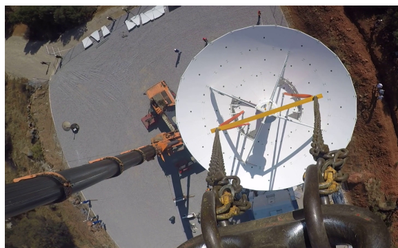
Fig. 3 The Big Lift—the VGOS telescope's azimuth cabin and main reflector being lifted and bolted onto the concrete structure.
