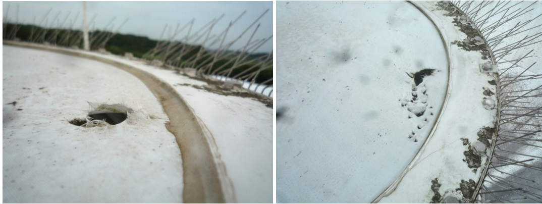
Fig. 3 A hole was found in the feedome sheet of the Kashima 11-m antenna in July (left). The hole was closed by tentative repair. However, additional holes were found in August (right).
