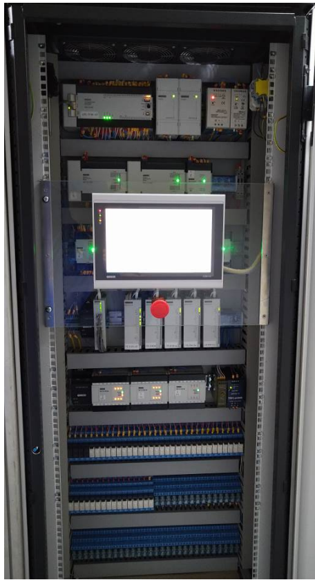
Fig. 2 General view of the DCS rack.
