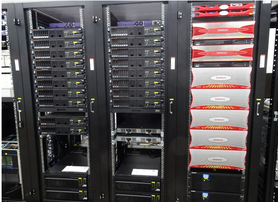
Fig. 1 View of the main system (data processing servers and storage) at the Tsukuba VLBI Correlator.
