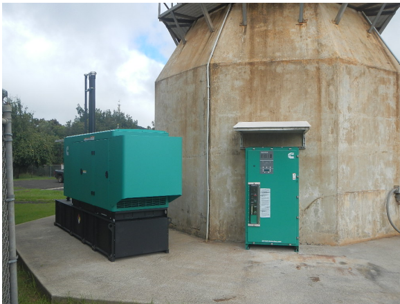
Fig. 4 New 20-m telescope 60-kW GenSet.
