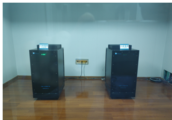
Fig. 6 The new hydrogen clock room.
