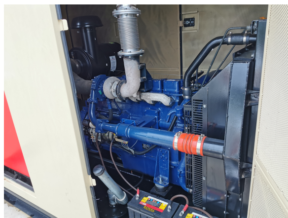
Fig. 6 Inside the housing of the VGOS antenna's backup generator.
