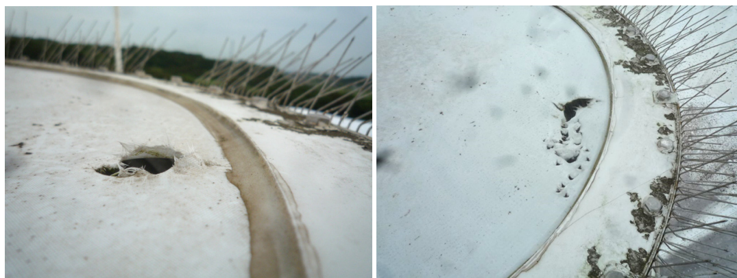
Fig. 3 A hole was found in the feedome sheet of the Kashima 11-m antenna in July (left). The hole was closed by tentative repair. However, additional holes were found in August (right).
