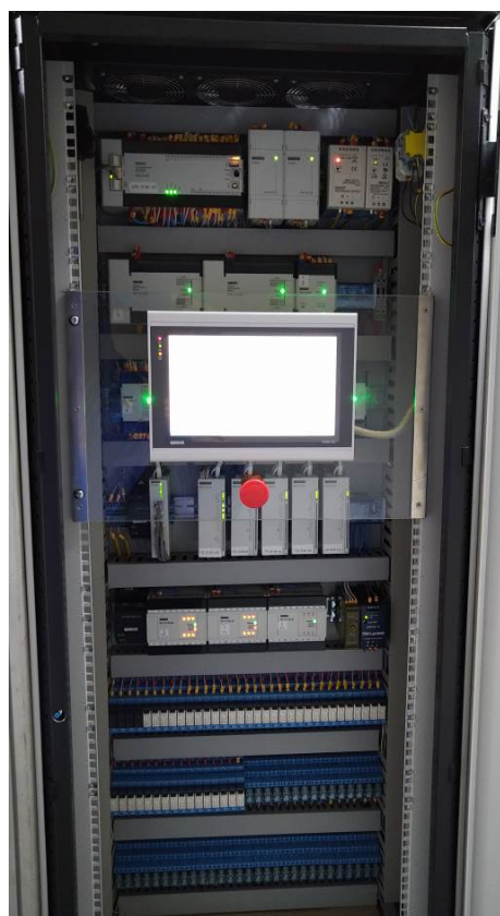
Fig. 2 General view of the DCS rack.
