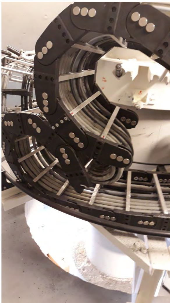
Fig. 3 Detail of the cable wrap structure breakage.
