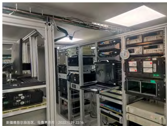
Fig. 3 The digital backend systems for VLBI and single dish operations, working in the walk-in electromagnetic shielding box under the telescope base.
