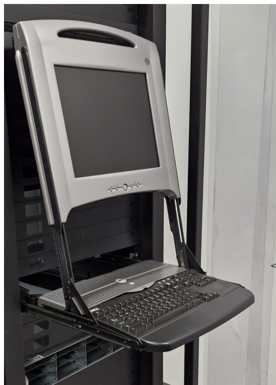
Fig. 2 Picture of new upload terminal in GA server room.
