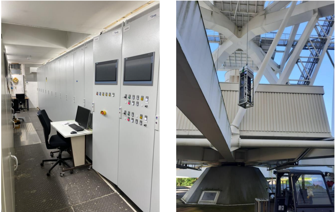
Fig. 2 Installation of the new racks in the telescope (photos by H. Homburg).
