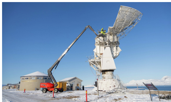
Fig. 3 A Norwegian company was contracted to finish the demolishing work in September 2023. (Image: Dag S. Roland)
