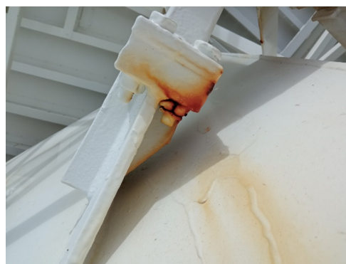
Fig. 8 Example of the status of the bolts in the back structure of the antenna.
