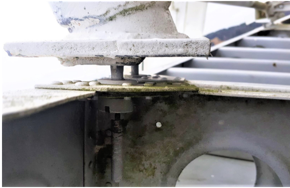
Fig. 1 The old panel and its fasteners.
