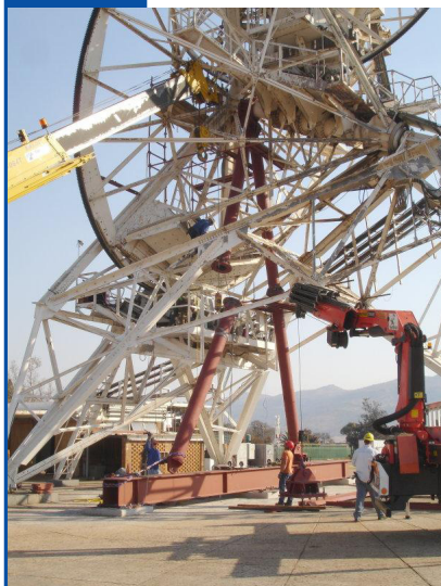
The legs of the custom A-frame support structure slot into place beneath the failed bearing housing. Note how the massive steel beam at the base acts as a bridge across the sub-surface tie-beams of the original antenna foundation.
