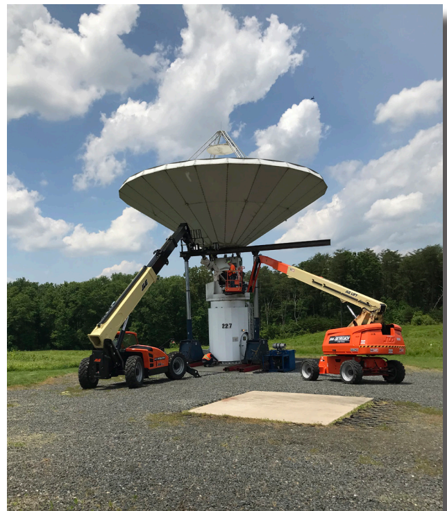
ISI technician inspecting the bottle jack and support beam installation prior to the jackscrew removal.
